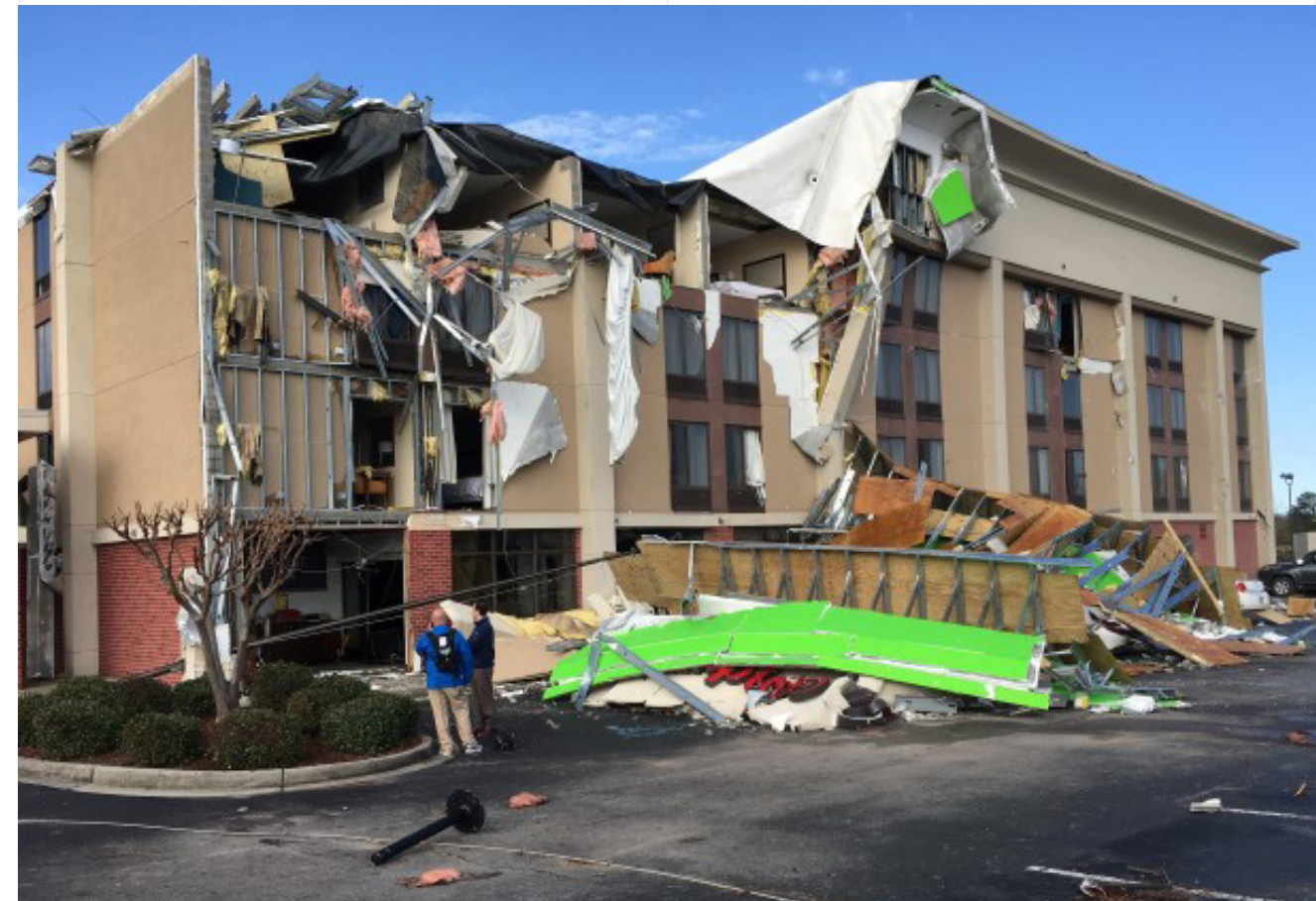
A Hampton Inn damaged by the tornado, photo courtesy of NWS BMX
